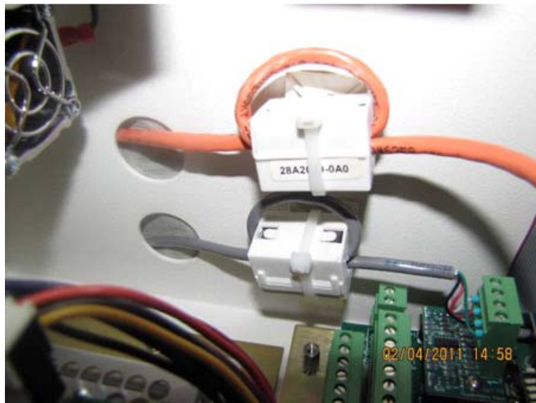
Figure 4.4b: Incoming I/O and Ethernet with ferrites installed
