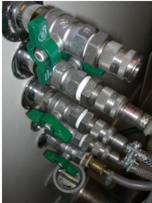
Example of valve:
